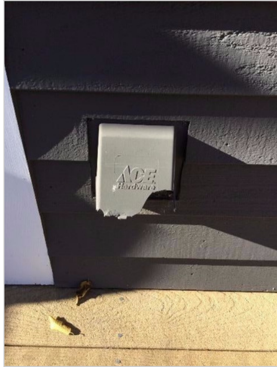
Cracked outdoor outlet cover should be replaced. Keeping moisture and water out of these outlets is important.
