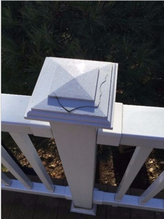
Crack in top cap of post. Non-structural - just visual impairment.
