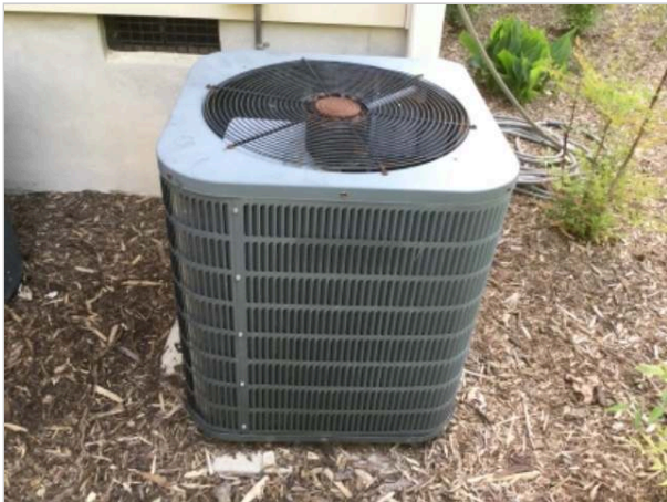
Right side outdoor unit
