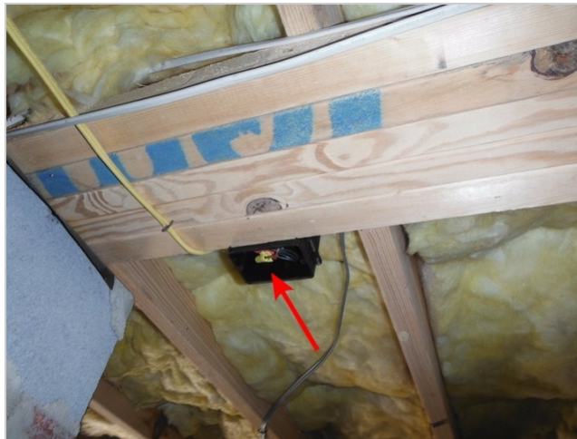
Open junction box-Crawlspace
