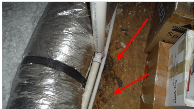
Deck staining below exhaust vent-attic
