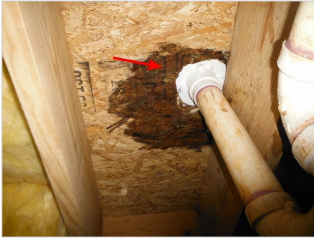
Staining/elevated moisture-Stall shower
