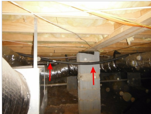
Water line not fully supported
