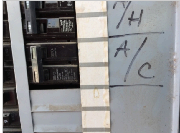
Circuit Breaker- 50 Amp
