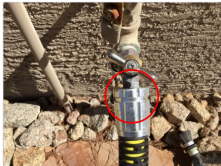
No Vacuum Breaker
