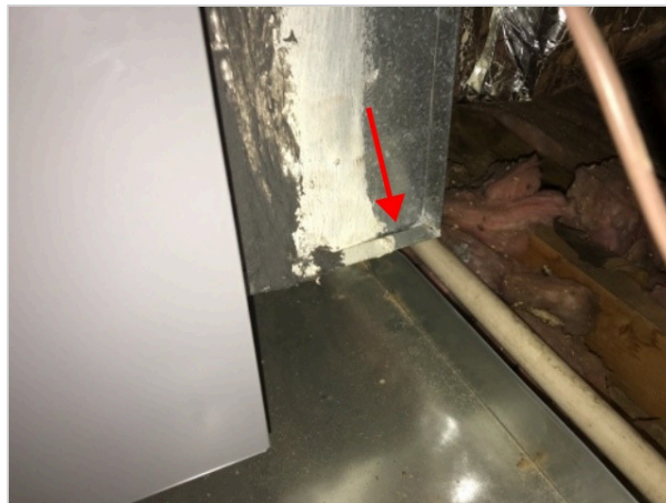
Right Side of Air Handler
