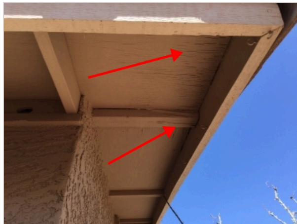
Front Left Corner
