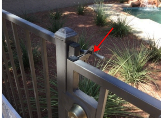
Gate Requires Adjustment
