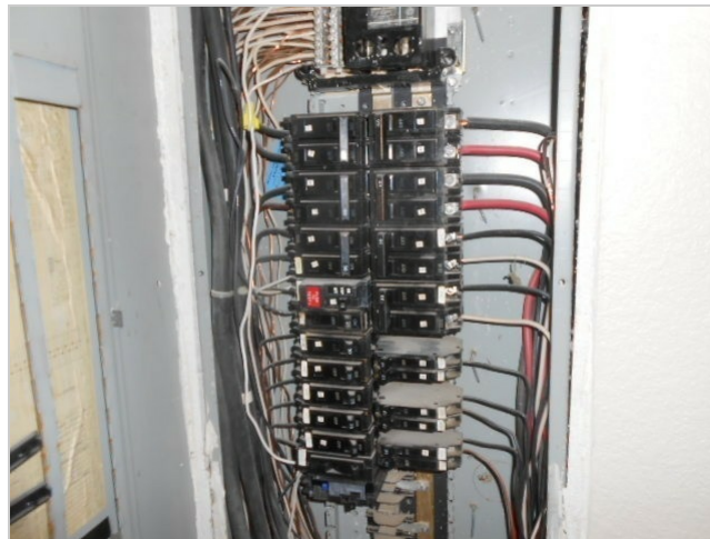
The electrical panel cover was removed for inspection of the house wiring, circuits and breakers.
