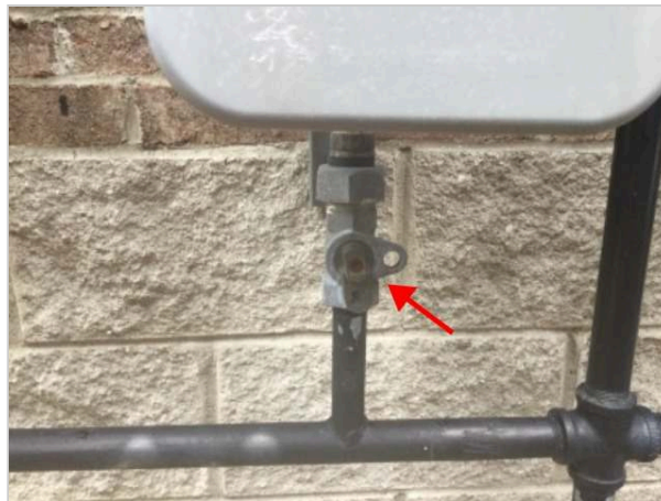
Main gas shutoff
