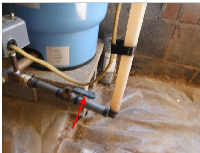
Water shut off-Crawlspace
