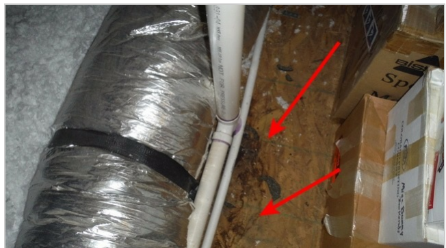
Deck staining below exhaust vent-attic
