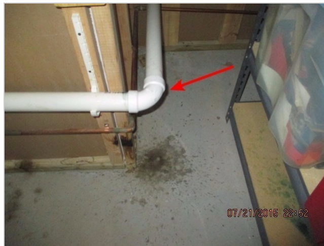
Bathroom sink drain line not glued and leaking
