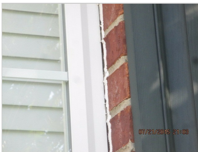
Missing caulk on front window
