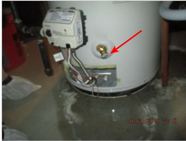
Leaking drain valve on water heater
