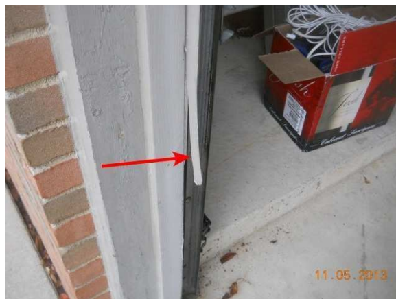
Damaged weather-strip(s) typical
