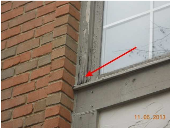
Peeling paint/deteriorated wood
