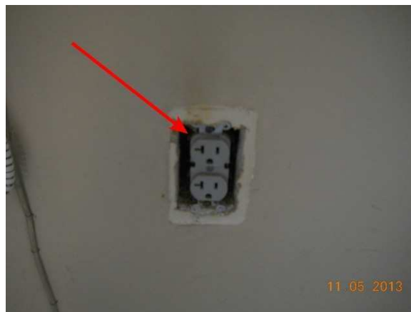
Missing cover (typical)
