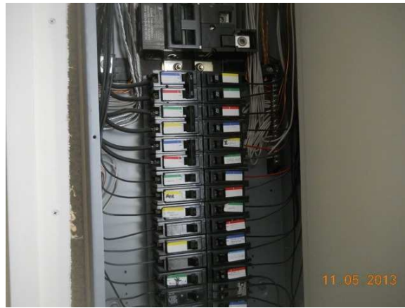
Panel cover missing
