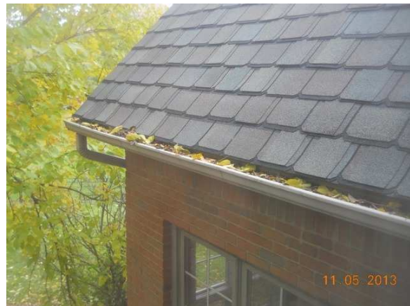
Gutters need cleaning
