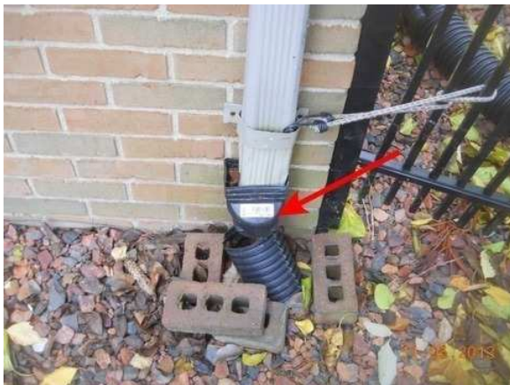
Not connected to drain
